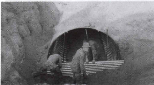
Combat Engineer support for the exercise was in heavy demand and provided by 4 CER. These photographs show the plant and operators constructing the underground Command Posts. During the exercise both the Ops, Pers/Log CPs and the RAP were underground.
